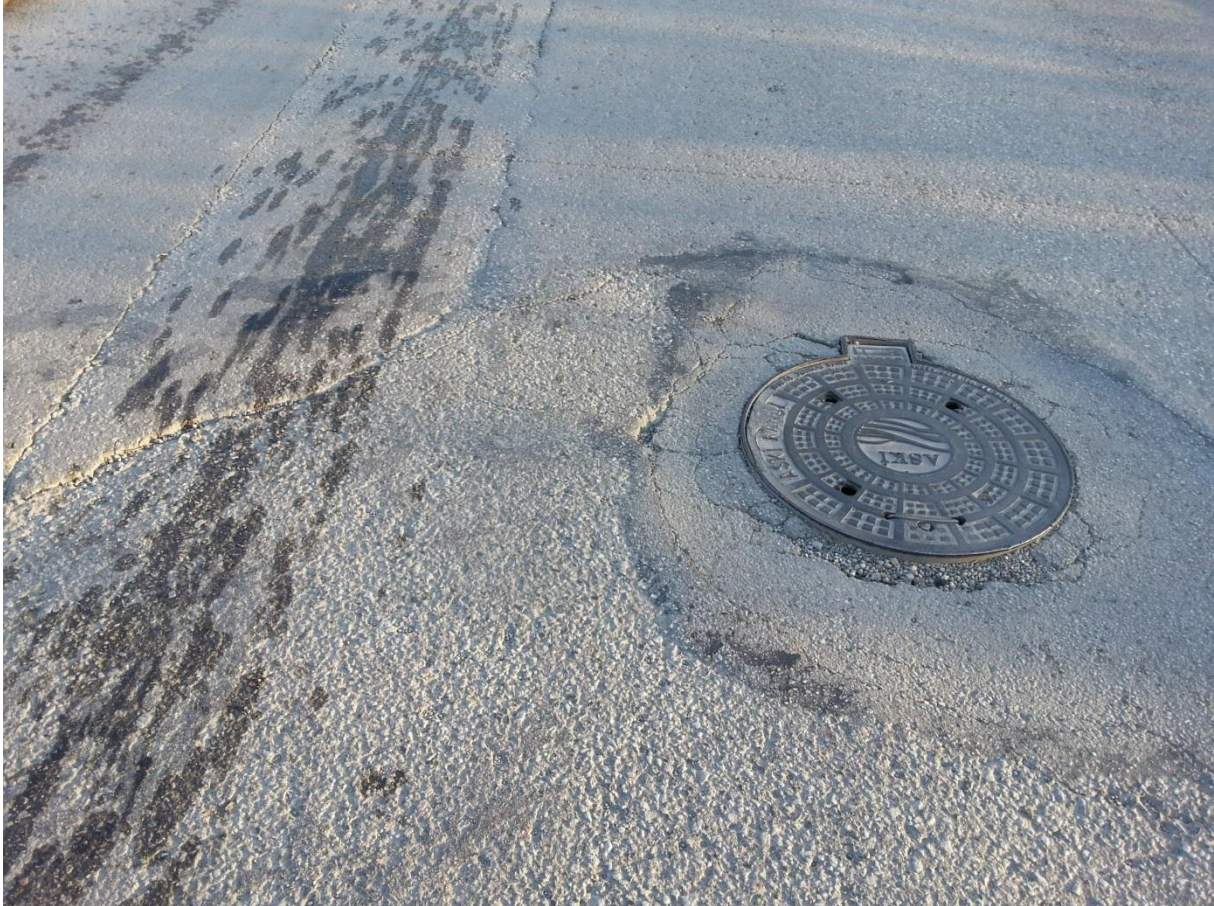
Figure 9 - Moderate Severity Patch Deterioration
