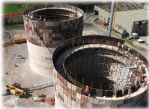
Figure 1: Overground Water Tanks
