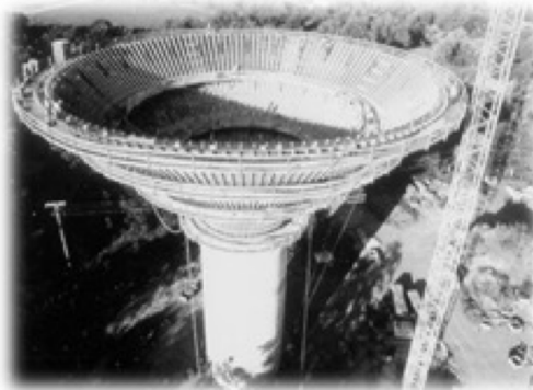
Figure 3: Overhead Water Tanks
